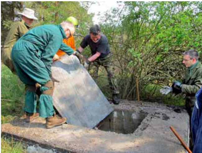
Opening up Cable Entry Shaft 3 required the removal of one of two original Metal Covers. Photo Clive Penfold
